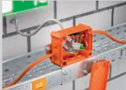
FireBox mounting with mounting plate on cable tray.
